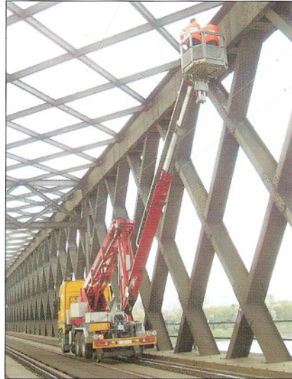
Even on railway tracks with aerial contact line, areas above the bridge deck can be reached save and easy.
